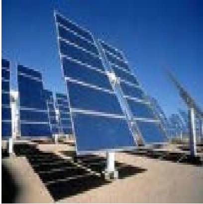
Solar electric panel
